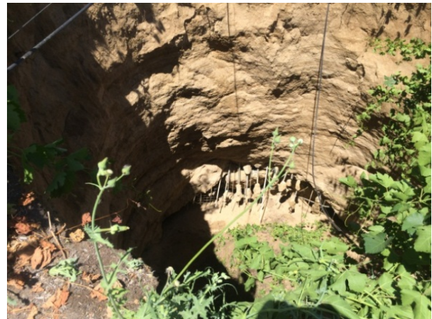
Figure 2b. Looking down into the tunnel; vine vegetation and wires from trellises on the surface fell into the opening.
