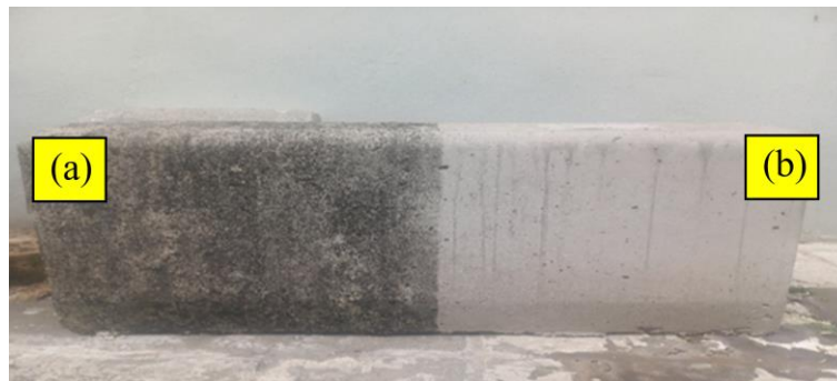
Figure 7. Visual appearance of concrete specimens after one year of outdoor exposure: (a) uncoated control concrete (CC) with visible moss and fungal growth, and (b) coated concrete (MFC) showing no biological contamination
