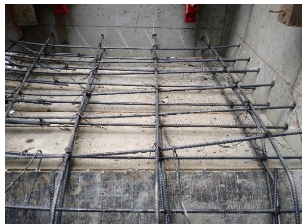
Figure 17. Negative slab steel, arched by the passage of workers
