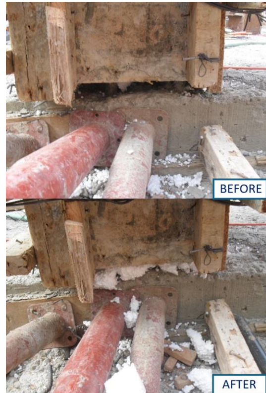
Figure 7. Incorrect formwork procedure at the base of a column
