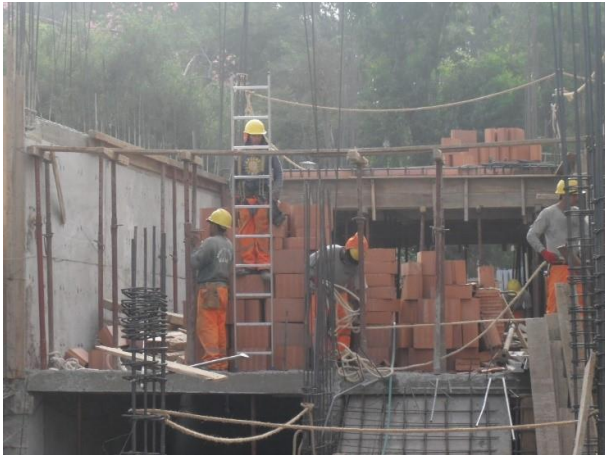
Figure 22. Excess ceiling bricks piled up on a slab
