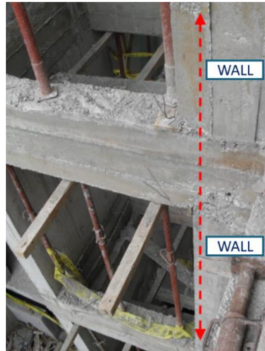
Figure 12. Structure that will house the elevator, with walls misaligned to the vertical
