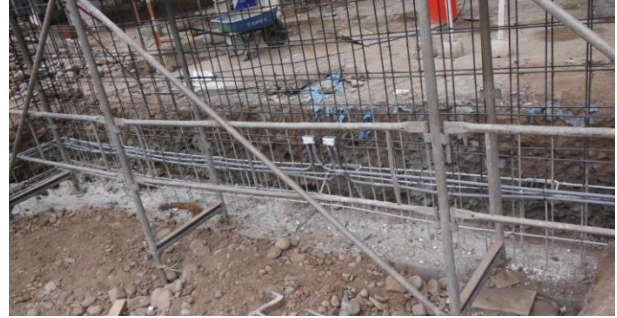
Figure 9. PVC pipes installed incorrectly and horizontally within the reinforcement of a reinforced concrete wall
