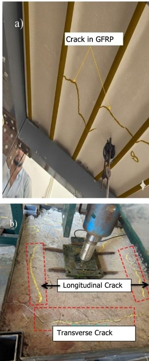
Figure 12. Crack Patterns a) Bottom of the slab, b) Top of the slab
