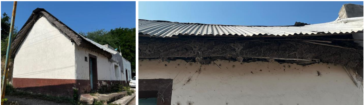
Figure 2. An example of a palm roof covered with sheet metal for enhanced durability. (Source: Photos were taken by the author)
