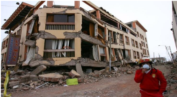
Figure 1. Building collapse due to accidental torsion effects during the Pisco earthquake, associated with the eccentricity between the center of mass and the center of rigidity
