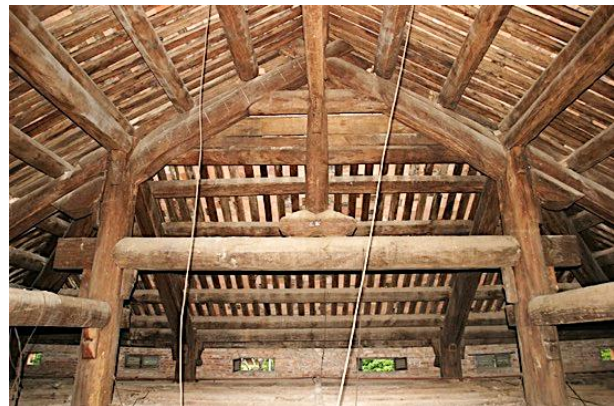
Figure 9. Upper wooden structure where the big beam, main tie beams, diagonal beams, and the columns work together
