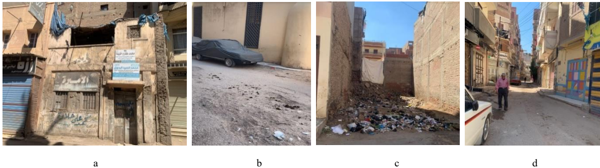
Figure 12. Dilapidated buildings in the third district, Ref. [researcher]
