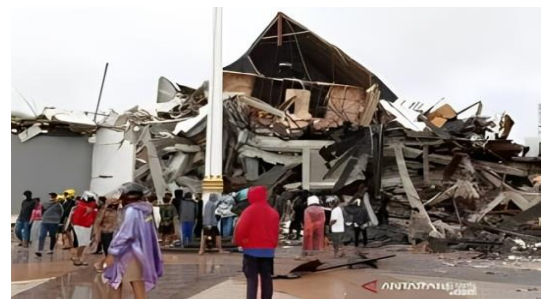
Figure 2. Severe Damage to the Structural Element of the West Sulawesi Governor Collapsed during the 2021 Earthquake
