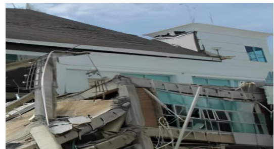
Figure 1. The West Sulawesi Governor's Office Collapsed During the 2021 Earthquake
