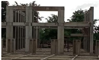
Figure 1. Utilization of Beams and Columns with RISHA in the Construction of Budibakti Elementary School
