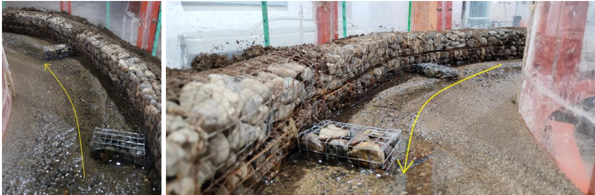
Figure 9. Sedimentation patterns observed upstream and downstream of Fin Gabion A, highlighting the deposition of sediment downstream of the structure
