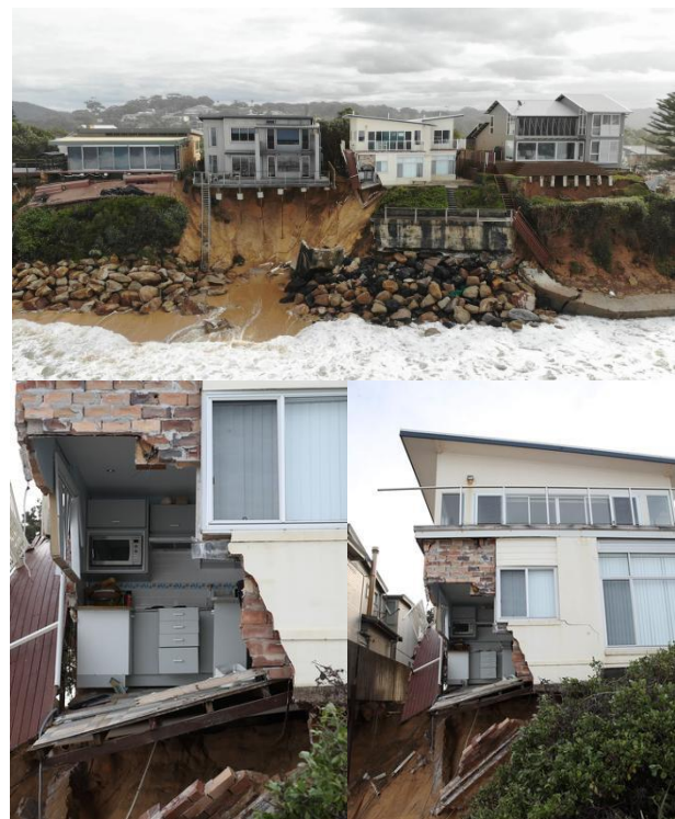
Figure 4. Images demonstrating the effects of coastal erosion on buildings in coastal regions [42]
