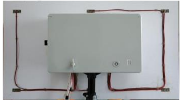
Figures 12. Electronic electrical control board
