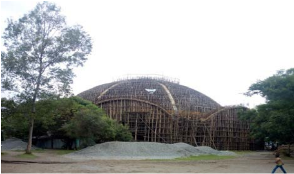
Figure 1. Eucalyptus vertical posts to prepare hemispherical dome formwork for St. Mary church under construction in Tikur Wuha town, Oromia, (Ethiopia)
