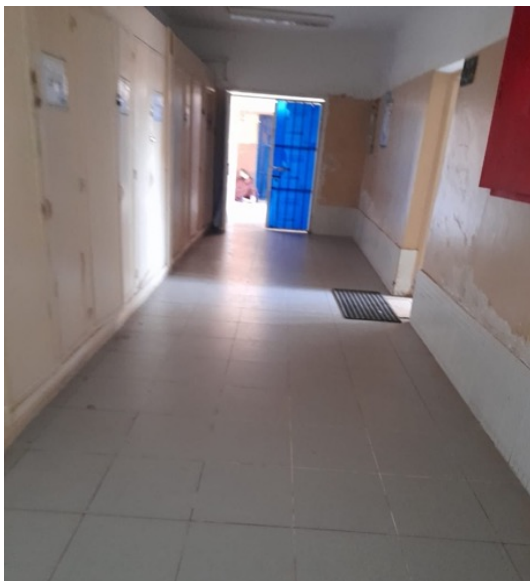
Figure 33. Inpatient Corridor with improper environmental quality - researcher
