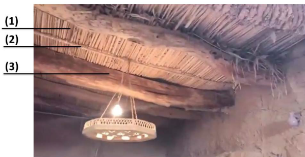
Figure 2. Traditional Date Palm Midribs and Thick Acacia Logs Using Habk Technique in Balat village. (1) Date palm midribs. (2) A thick date palm midrib as Hommar. A date palm leaflets ropes, Shalaq, is used in tying Hommar to the midribs. (3) An acacia log beam
