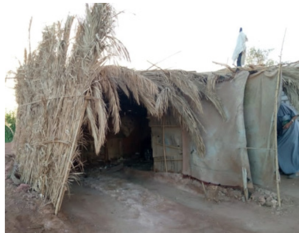
Figure 9. A garage made from leaves and cardboard in new Qasr town from the inside. (1) leaves in the roof of the garage. (2) Cardboard sheets. (3) midribs lattice. (4) leaves outer wall
