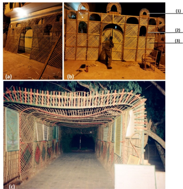
Figure 12. Gate made from PMP. (a) The panel before installation. (b) The panel after installation onsite. (c) Shaded pathway made from PMP. (1) Arched midribs ornaments. (2) Timber frames. (3) Diagonal midribs nailed to the timber frame
