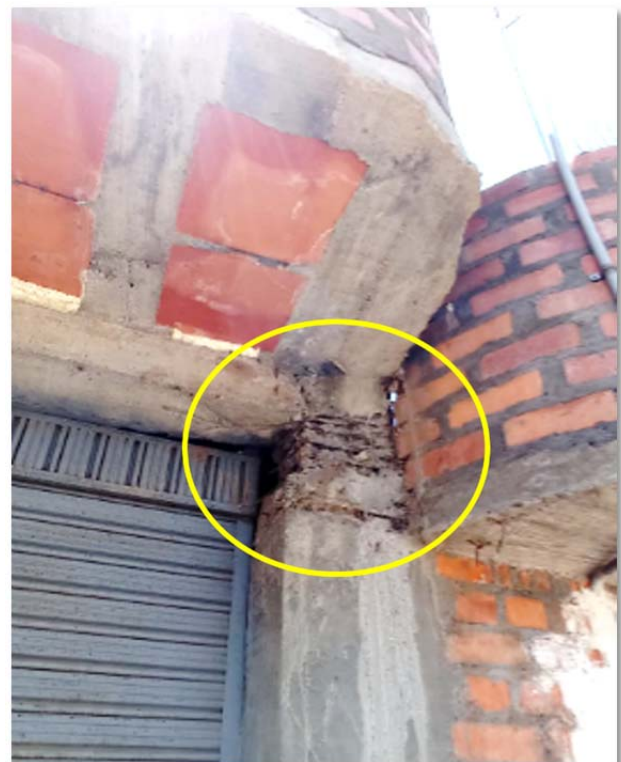
Figure 9. Reinforcing steel exposed to corrosion
