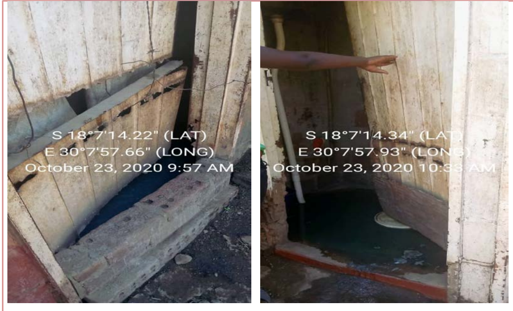
Figure 4. Toilets/Sanitation situation in Kaguvi
