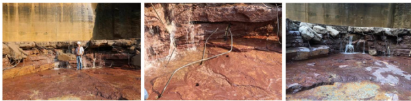
Figure 1. Corrosion damage at stepped ramp
