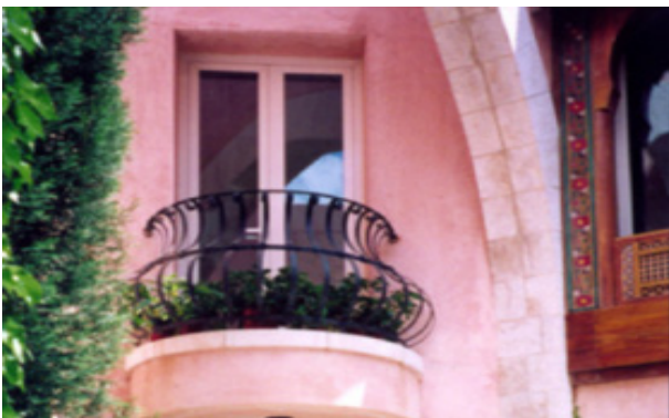
Figure 7. Al Tabbaa Villa: Safety and security had been achieved using different features such as railing.
