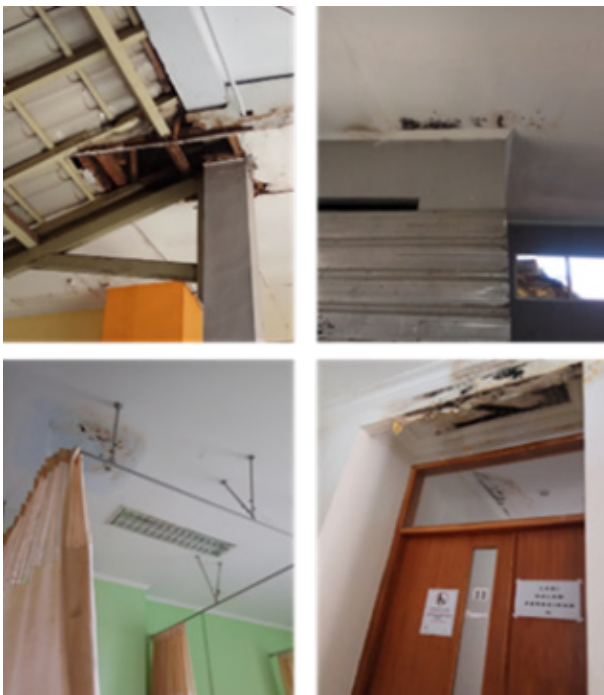
Figure 4. Ceiling damage photos
