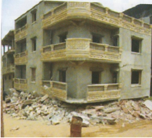
Figure 7. Destruction of a building with a flexible first floor during the earthquake in Boumerdes (Algeria, 2003) [Nemchinov, 2008]
