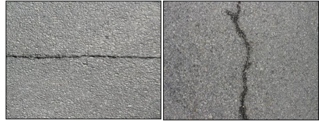
(a) Transverse crack
