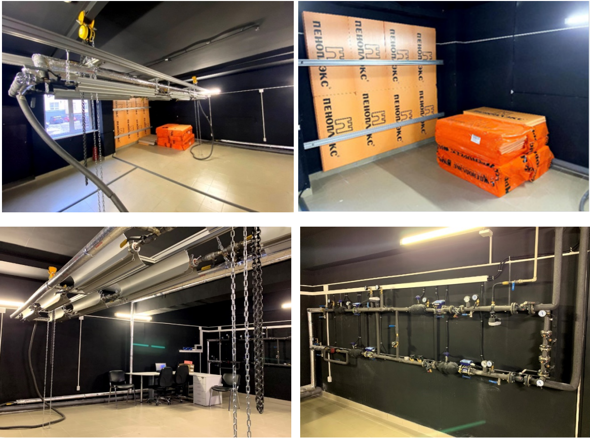
Figure 2. General view of the Radiant Heating Laboratory
