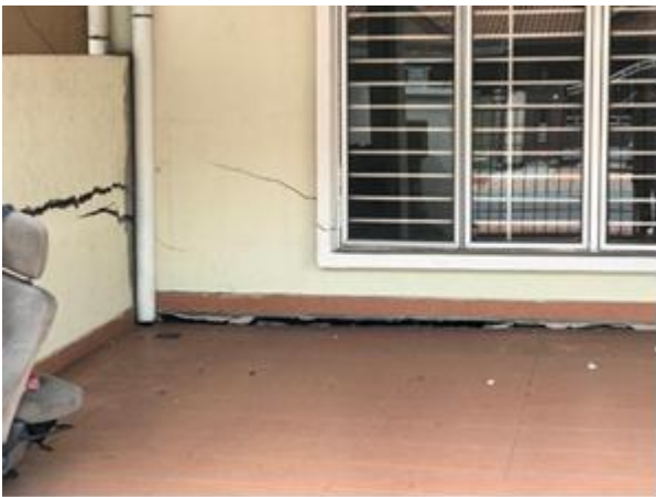
Figure 7. Neighboring house was experienced visible deflection of the floor ground slab and cracks on wall due to soil settlement.
