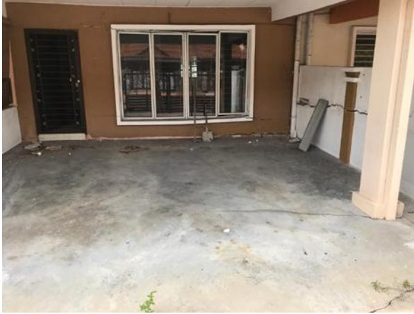
Figure 6. Structural damages with visible cracks were observed in front of house under study with structural and non-structural components.
