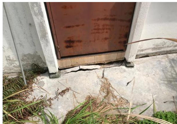
Figure 12. Splitting between ground floor and wall
