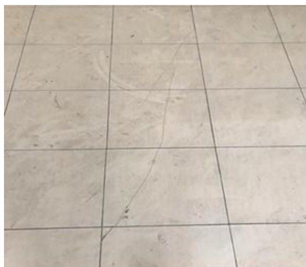
Figure 13. Cracking on the tile and floor
