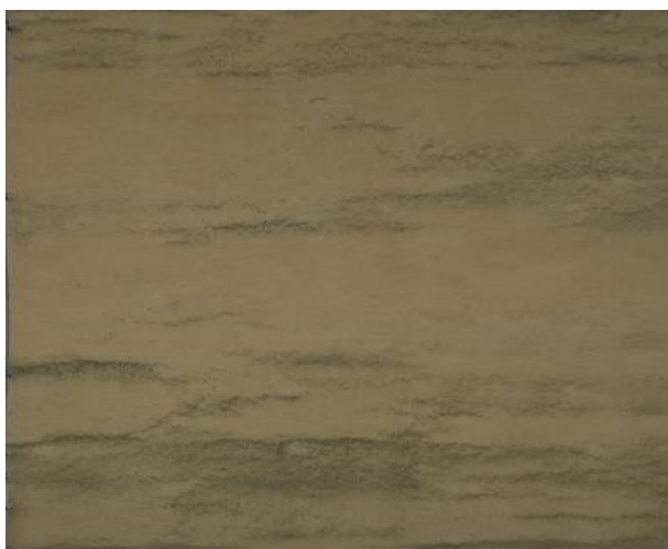
Figure 8. Exterior facade of a prefabricated panel type block of flats degraded by microorganisms [15]
