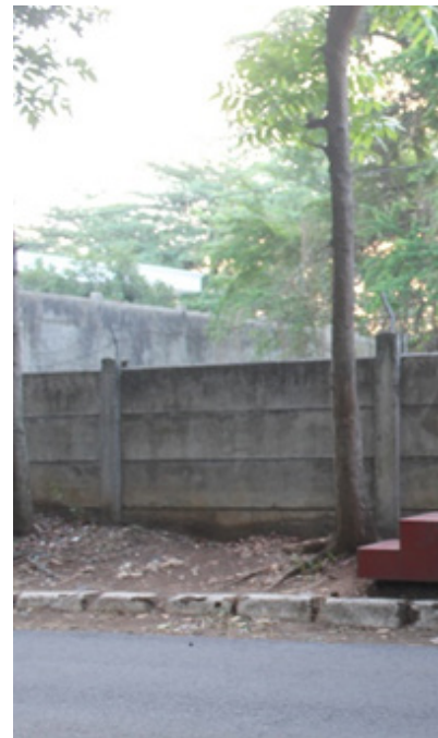
Figure 3. Condition of no leading pavement
