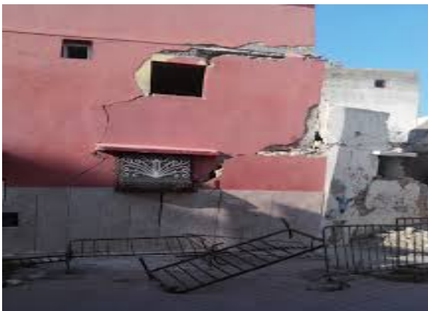
Figure 1. Photo of buildings threatened with collapse by an old fabric in Casablanca
