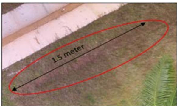
Figure 7. Tension crack of the slope
