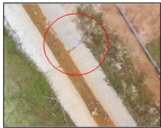
Figure 8. Lateral crack on surface drainage
