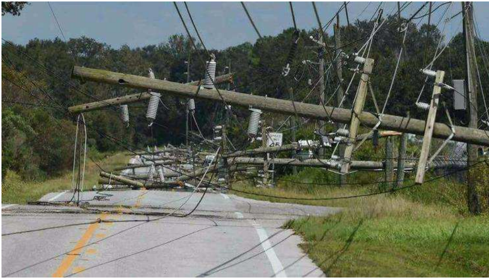
Figure 1. Downed power lines following Hurricane Irma [14].
