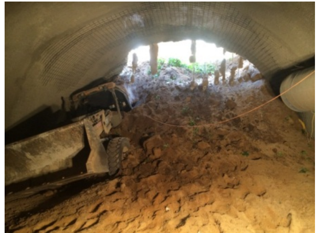
Figure 2a. Looking at sand fallout along tunnel bearing.
