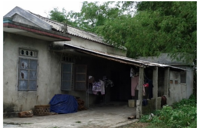
Figure 9. Local residents' home with broken windows and molded concrete wall
