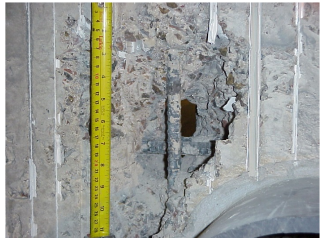
Figure 4. Poor concrete installation in Iqaluit wastewater treatment facility made the facility unusable.
