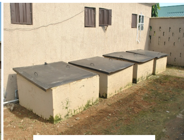
Primary treatment pit
