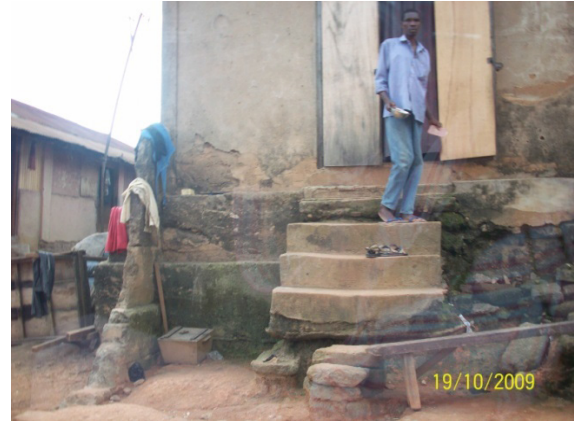
Plate 8. Dilapidated residential unit
