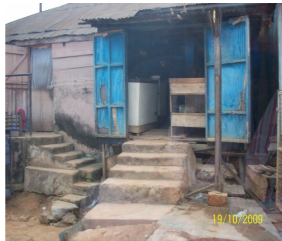
Plate 9. Dilapidated residential unit
