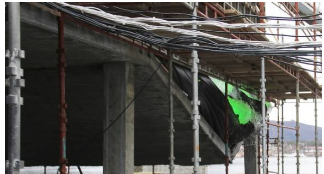
Figure 4. Test slab at the moment of collapse [20]
