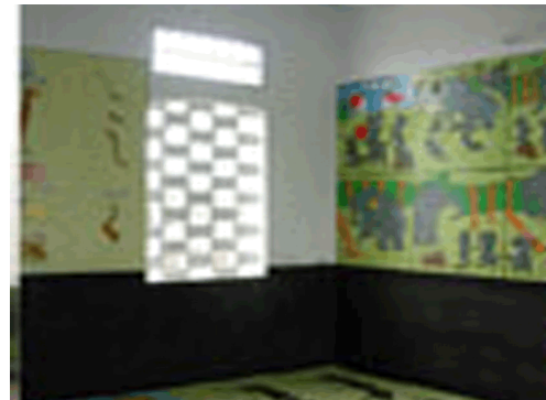
Figure 22. Classroom interior shows the brick lattice's window (DesignShare: Designing for the future of learning 2013)
