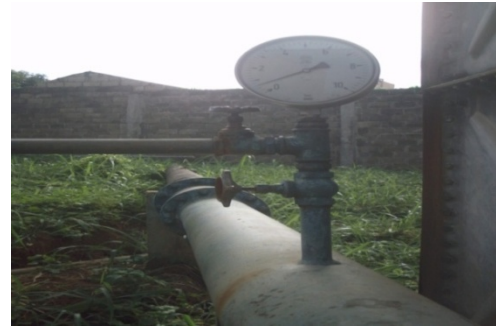
Figure 6: Gauge Meter for the Water Treatment Plant
