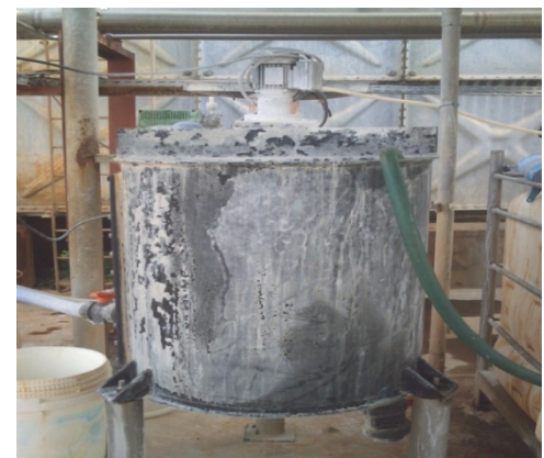
Figure 7: Pasteurizers and Water Treatment Plant
