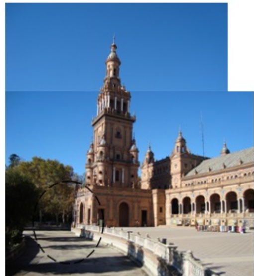
Figure 1. The plaza now without water (see above) and before with water (see left) scaffolding showing the damaged part
