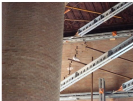
Figure 4. Crack of more than two inches appeared
