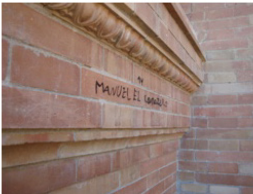
Figure 7. Texts on the walls need to be cleaned
