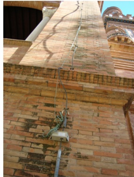
Figure 8. Bad electric wiring
