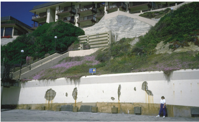
Figure 9. The Damages of Built Seawalls
